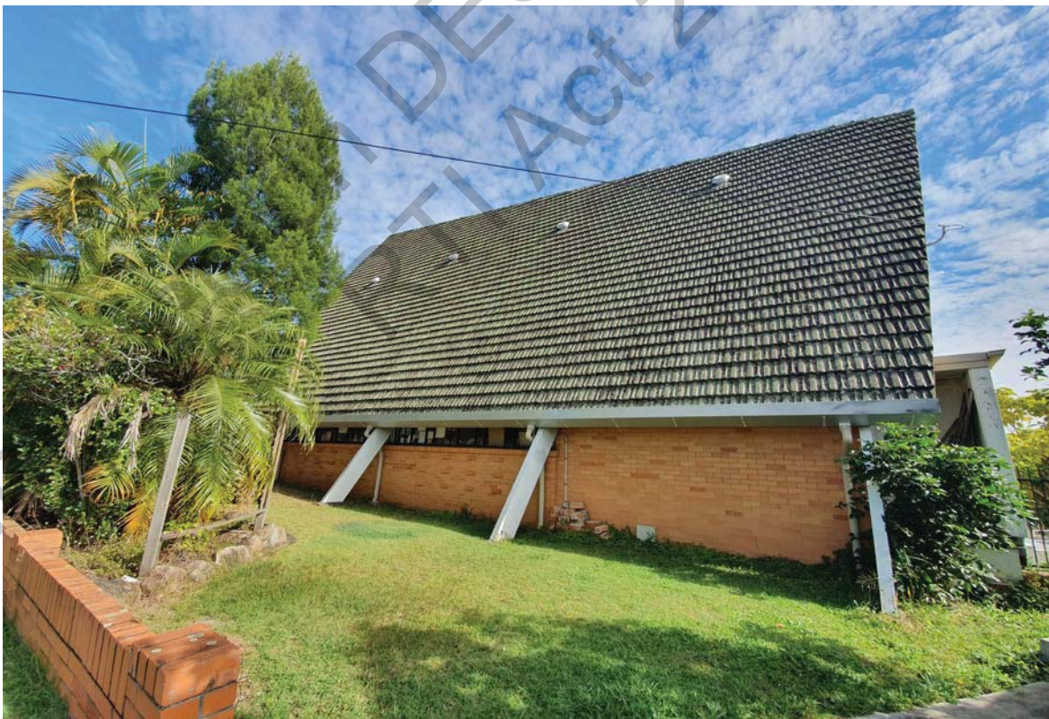
Figure 4: Southeast side of Church showing portal frame extending below eaves (Queensland Government, 2021.)
