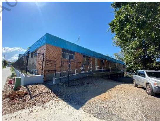
Figure 8. South Eastern corner of building showing ramp access to rear of building.
