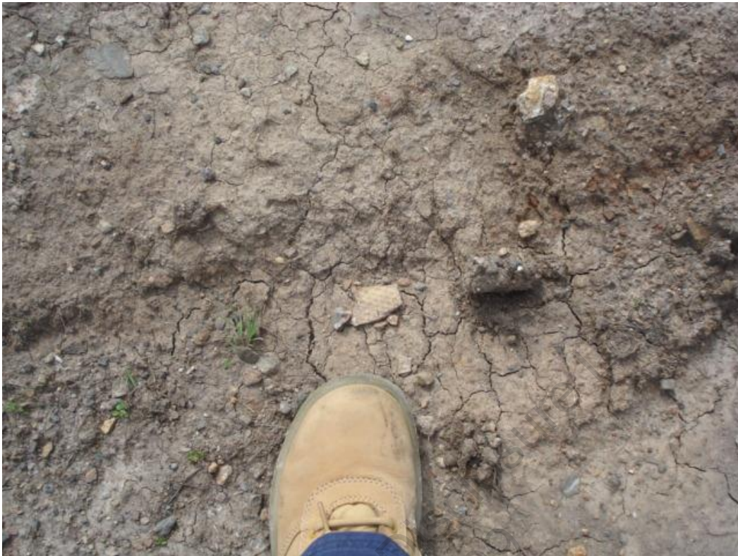
Plate 5 – Bonded (non-friable) ACM identified during field screening at TP06. Date: 01/04/2021
